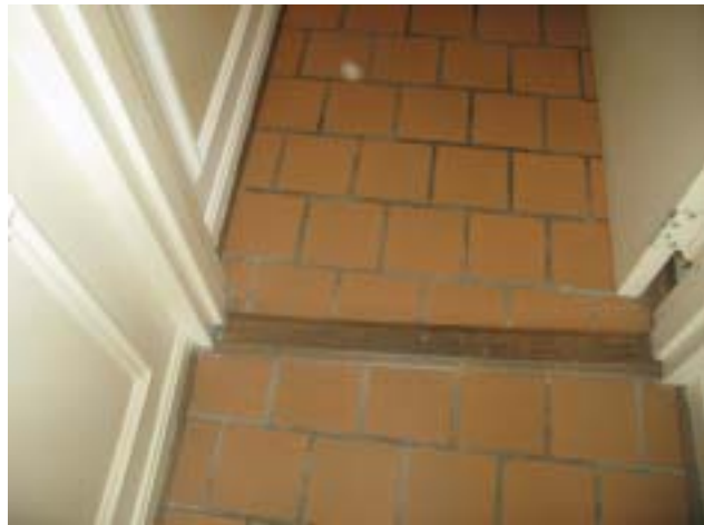
Wood threshold under the unit front door is loose to the floor. (safety) Needs to be secured.
