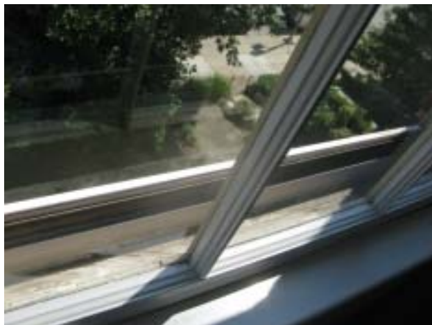
Glass putty is flaking off window sashes. Re-glazing and paint needed.
