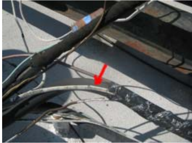
Electrical cable that provides power to roof mounted condenser unit has damaged outer jacket. (safety) This wire needs to be replaced.
