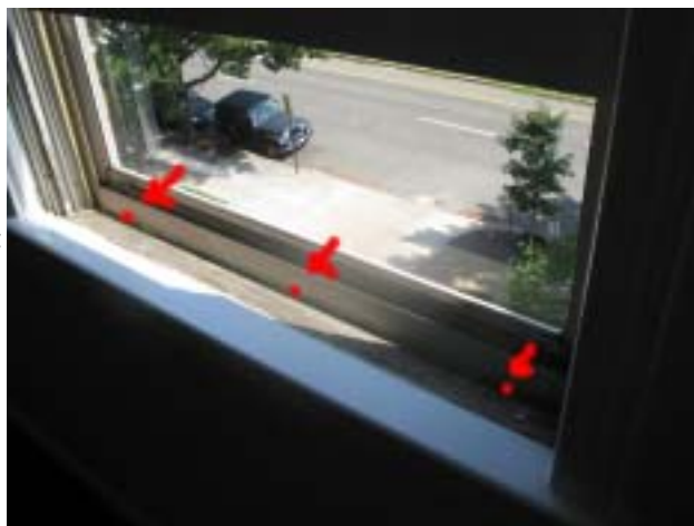
All storm window frames need drain holes added. All original sills need to be painted.
