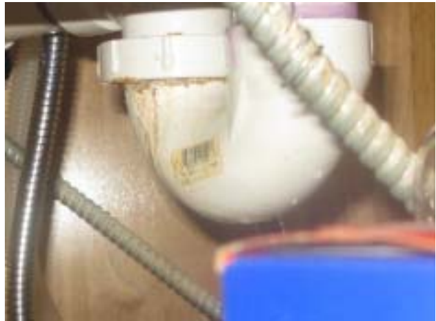
Signs of past leaking at sink drain assembly. No dripping at inspection.
