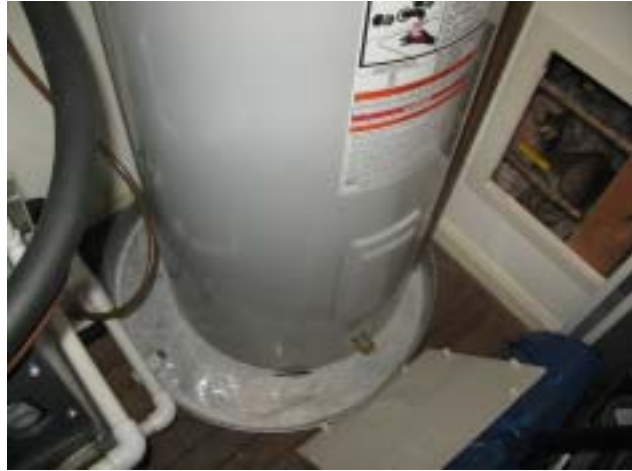
Safety leak pan installed but pan not connected to a drain. Will not serve function.
