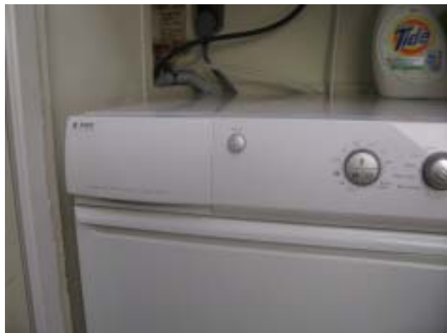
Clothes washer was not operational. Repairs or replacement needed.
