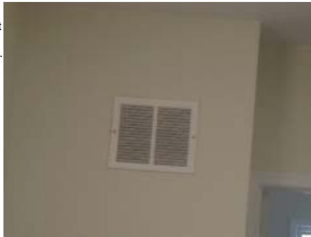
The top level return register is not designed to accept a filter. No filter installed. Repairs needed.
