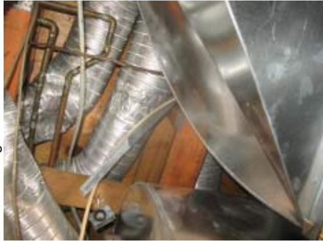
Small view of floor structure seen in the air handler room ceiling.
